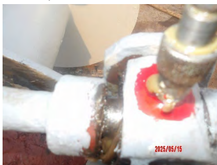
15 May –during greasing: brake spindle greasing point
