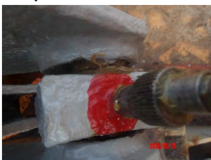
15 May – during greasing: brake band joint 3
