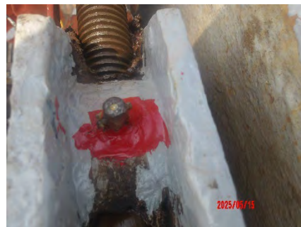
15 May – After greasing: brake spindle greasing point
