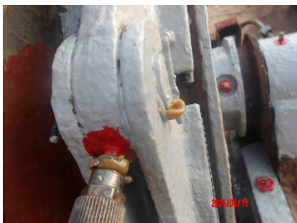
15 May – during greasing: brake band joint 1
