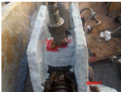
15 May –during greasing: brake spindle greasing point
