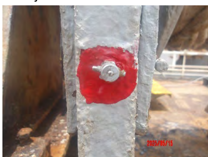
15 May – Before greasing: brake band joint 2
